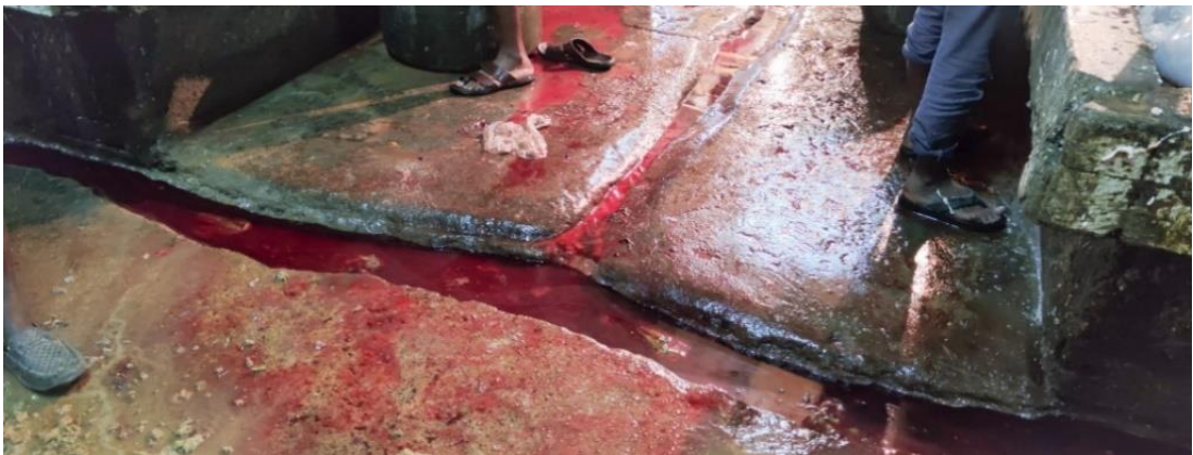
Pic- 4.10: Drainage system of a slaughter-house.
